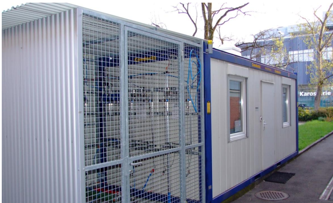
Figure. Test bench electrolyser at EMPA
