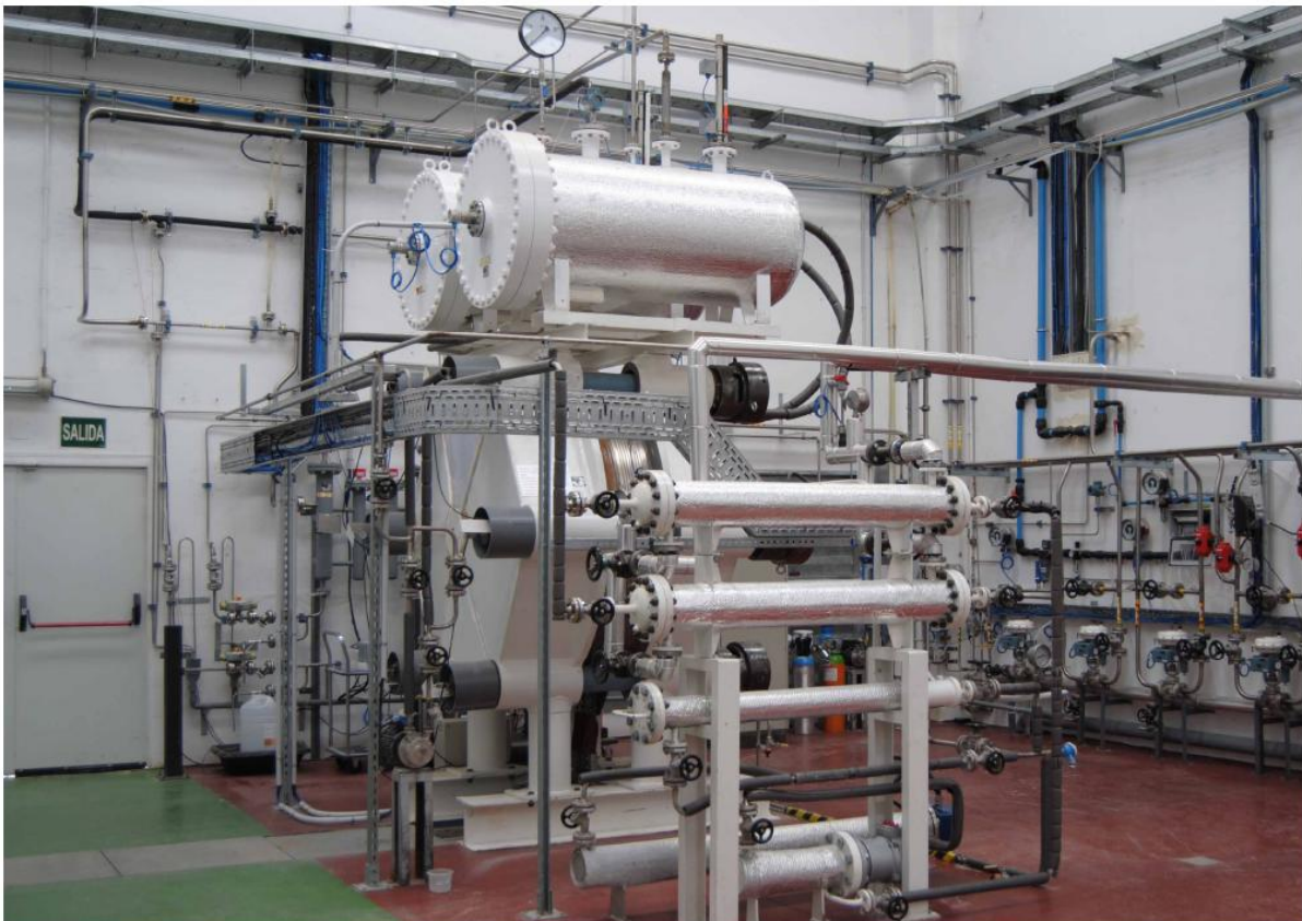
Figure: Picture of the electrolyser of IHT at FHA facilities
